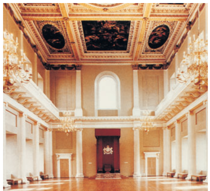
A covert Aspirated Smoke Detection System installed in the Banqueting Suite, Whitehall.
