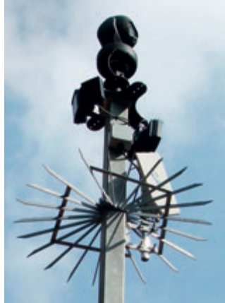
MoD training centre in South East England where Philton installed the very latest technology including IP based CCTV system which incorporates both conventional and IP cameras and is used for both security and training.
