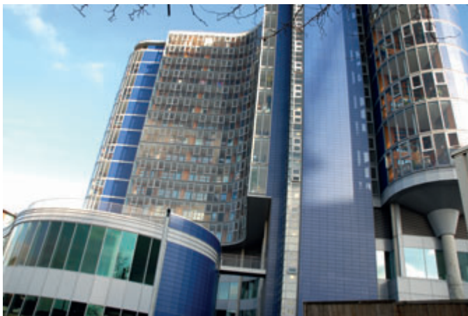
A networked Gent Vigilon Detection System installed at Falcon Wharf, London.
