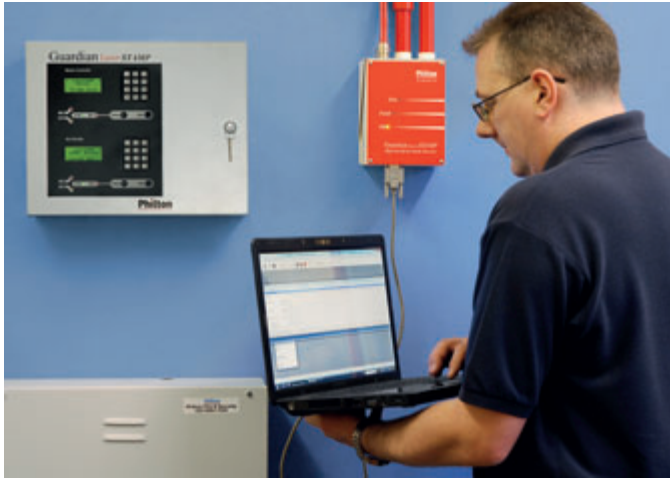
Guardian LaserSTAMP Aspirated Smoke Detection System, control panel and smoke detector.
